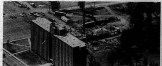
THE SECOND OF A COMPLEX OF FOUR residence halls planned for the eastern side of the campus, this dormitory for women will house 396 Murray State coeds when completed next year.
